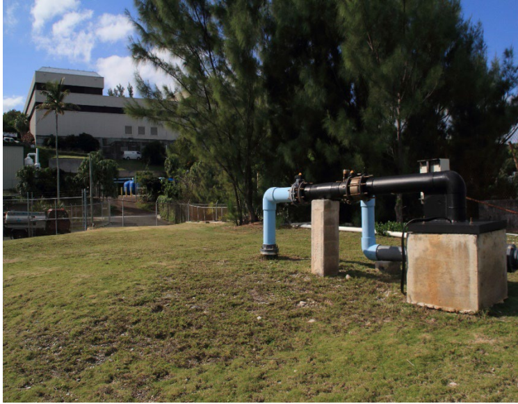
Seawater extraction well at Tynes Bay SWRO plant, SWRO plant and incinerator Plant in background, Incinerator is behind trees
