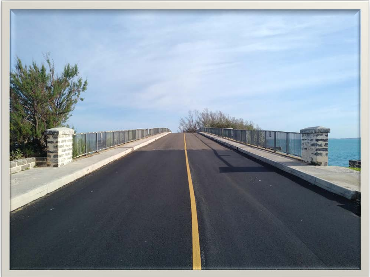
Figure 1 : Watford Bridge Looking North, Handrails to be Painted
