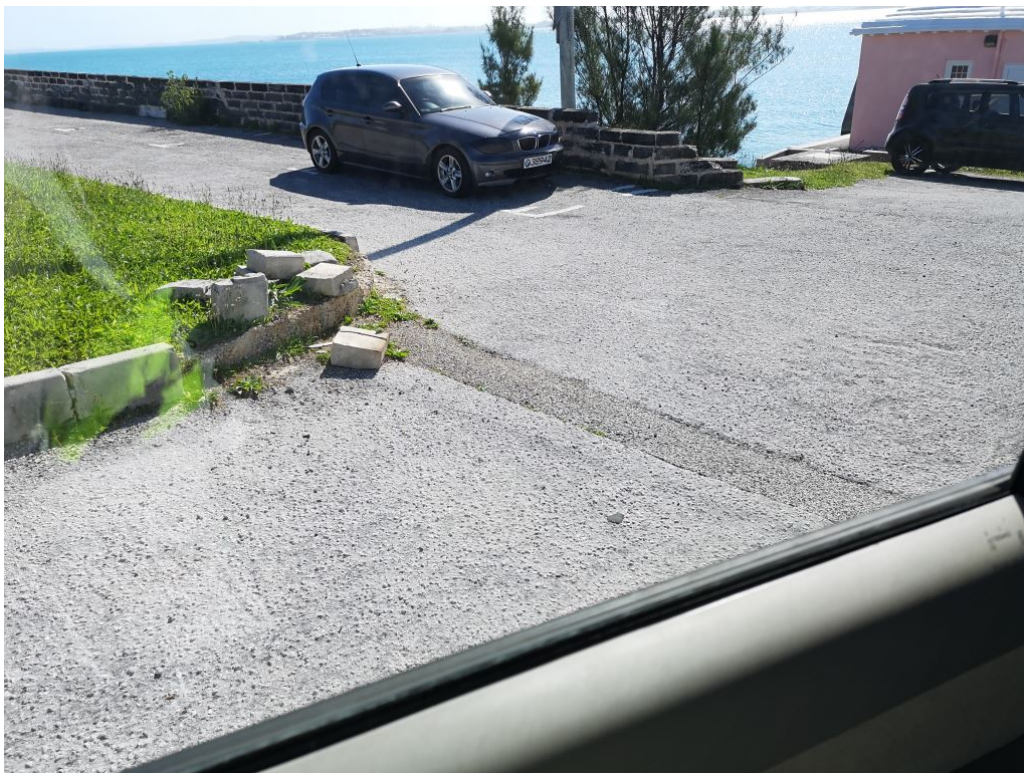
Figure 2. Additional broken kerb near Watford Bridge Ferry Terminal
