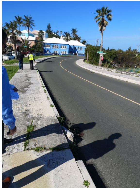
Figure 1. Broken kerb on West side of bridge
