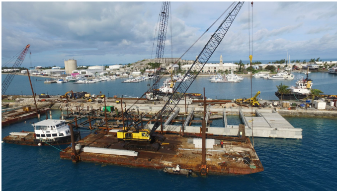
Figure 8. Local contractor working on the $15m Kings Wharf Rehabilitation project in March 2019
