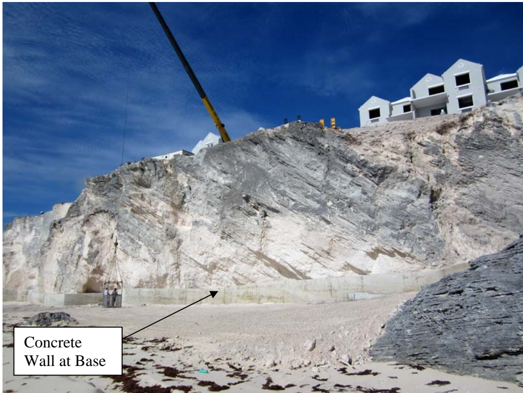
Photo 3: Eastern Part of Shore Cliff
