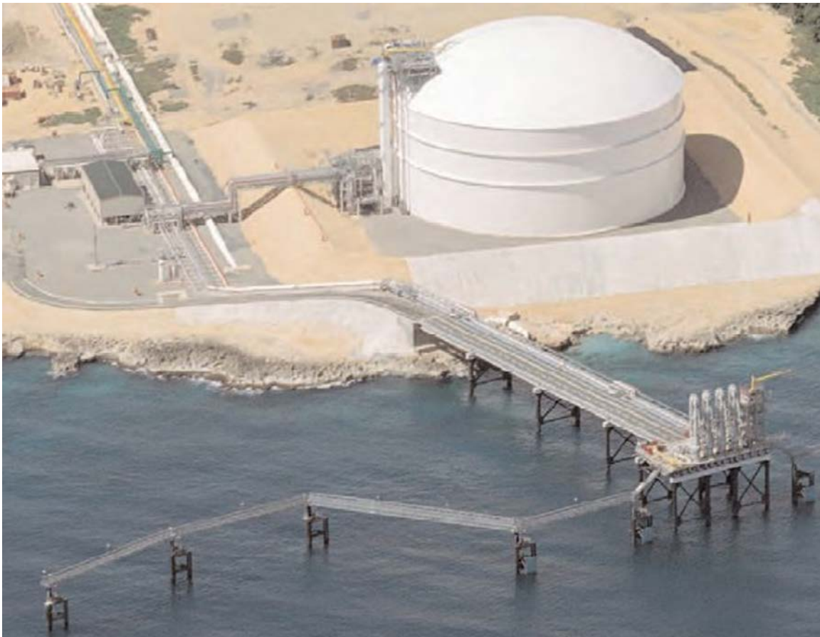
Figure 5.5: Re-gasification and Storage Facility
